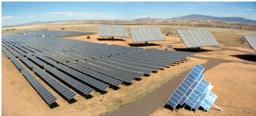
Photo 4 – Utility Large Scale PV Generation System
