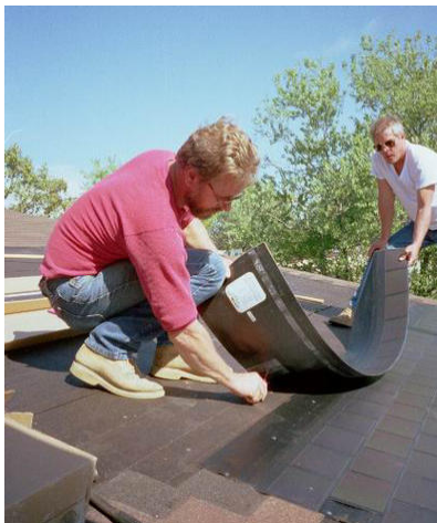
Photo 2 – Thin Film PV Integrated into Roof Shingles
