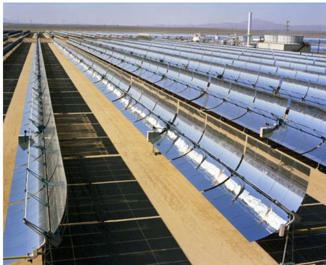
Photo 6 – Utility Scale Solar Parabolic Trough System
