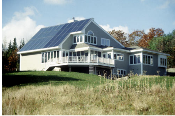
Photo 1 – Residential Silicon PV Application
